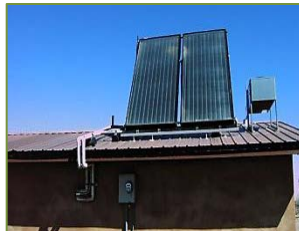
Solar Water Heater – Bosque del Apache
