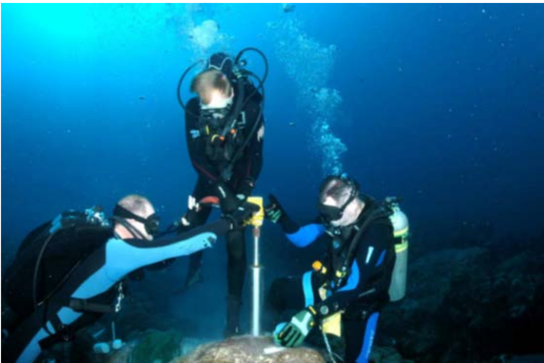
Figure 3. Divers use a coring drill bit to drill into dead reef rock to install a mooring buoy anchor.
