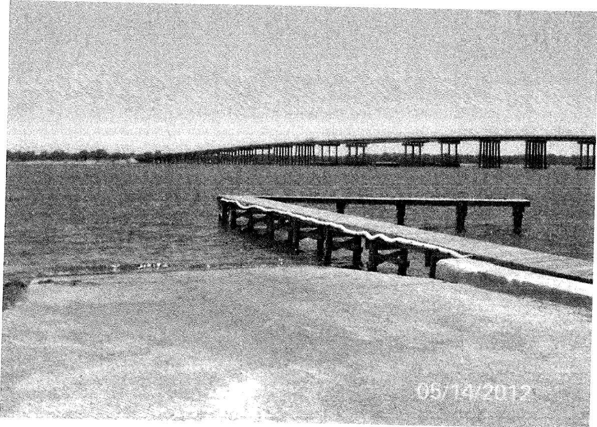
Figure 7. Photo of the proposed project area including the boat ramp and dock that will be repaired as part of the Earl Gilbert action.
