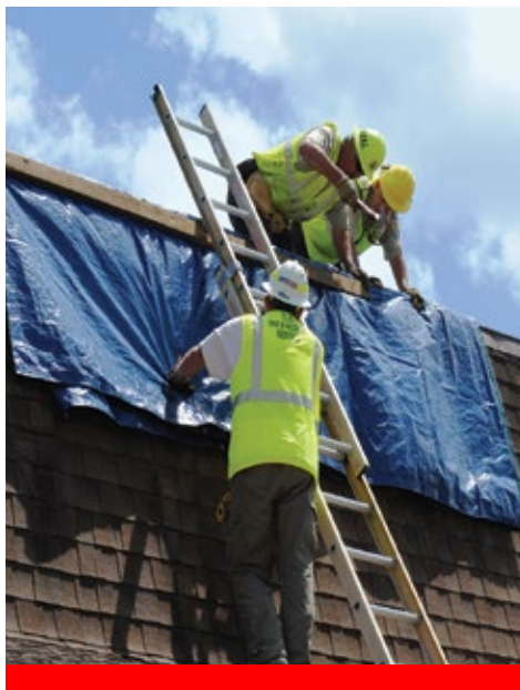
At Big Cypress National Preserve, U.S. Fish and Wildlife Service workers helped out their partners, the U.S. National Park Service, by nailing tarps down on three damaged roofs.
