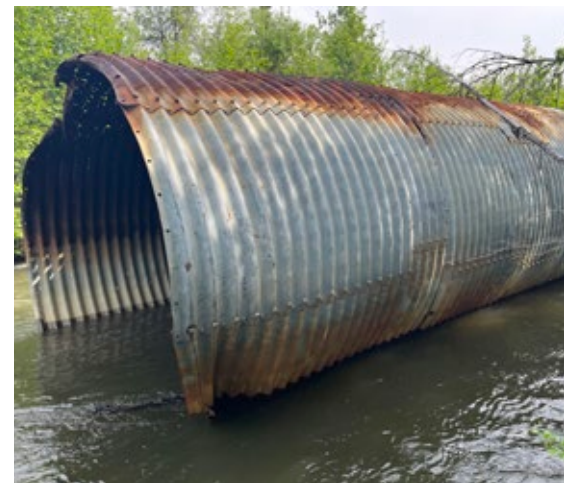
One of the undersized culverts that was carried downstream during a 2006 flood event on the Little Tonsina River in Alaska. (PHOTO BY JACOB MILLS/ALASKA DEPARTMENT OF TRANSPORTATION)
