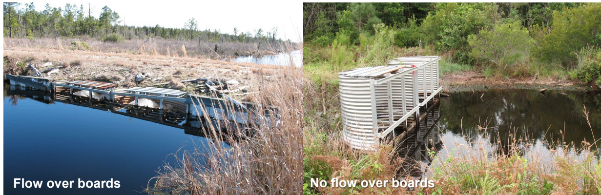
Figure A-12. Risers with water flow and with no flow over the top of the boards.
