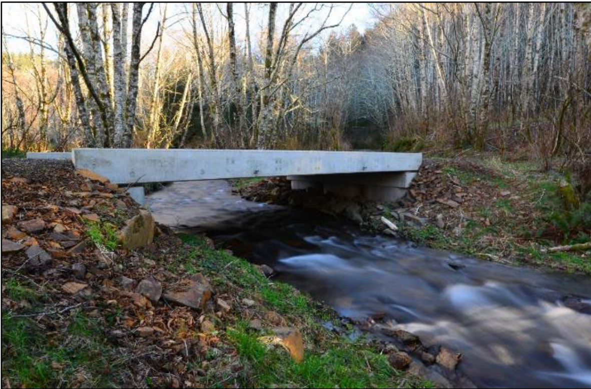
Photo (above): Restored fish passage in the Nestucca Basin along Oregon’s coast (credit: Scott Wright, River Design Group, Inc.)
