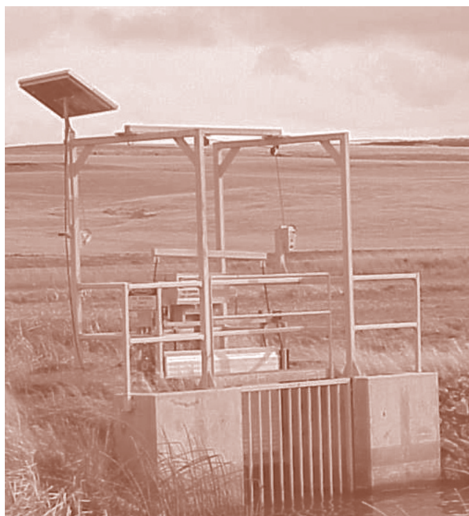
Bridge Creek Solar-powered Fish Screens, USFWS
