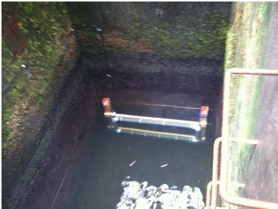
Figure 5. PIT antenna inside the lower fish ladder on Eagle Creek.
