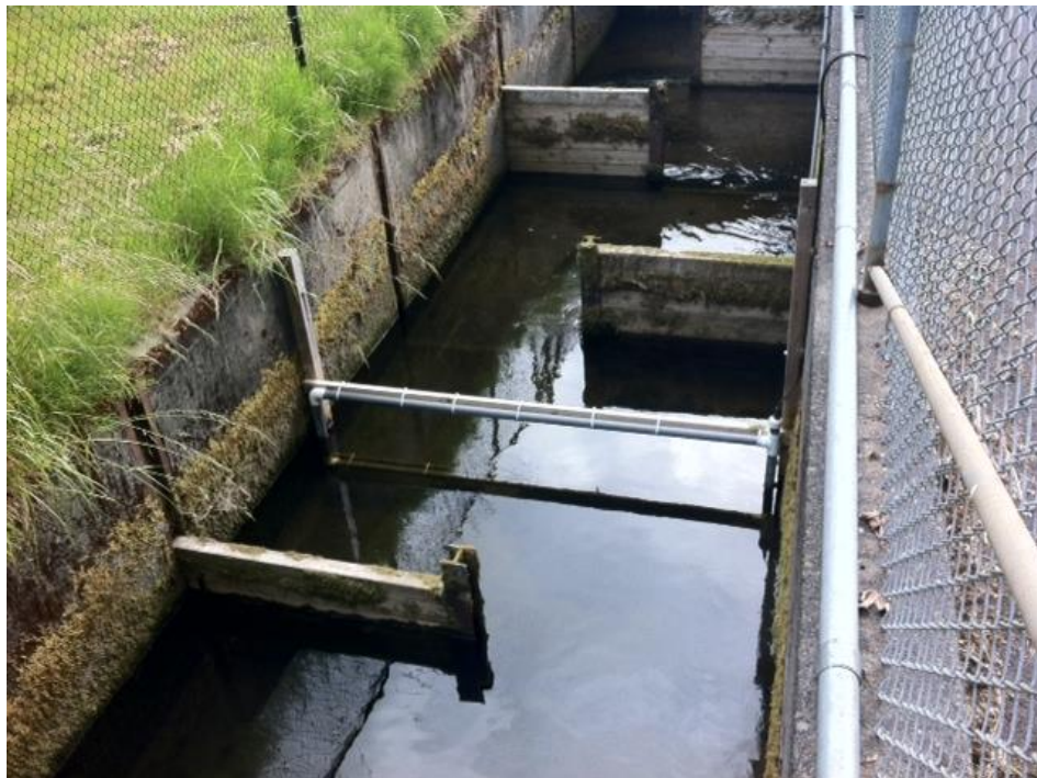
Figure 6. PIT antenna inside the hatchery fish ladder on Eagle Creek.
