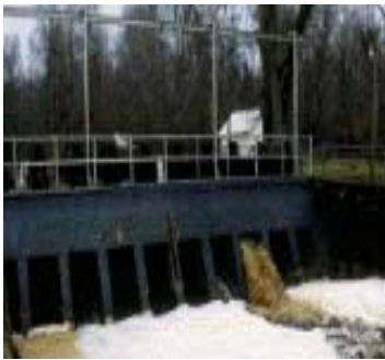
Lake Drummond Spillway. Water control spillway releasing into the Feeder Ditch. USFWS.
