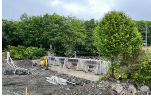
Replaced Diversion Dam and Fish Barrier at Makah National Fish Hatchery (Clallam Bay, WA); USFWS
