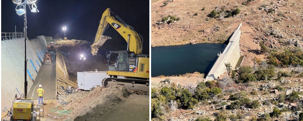
Comanche Dam during and after rehabilitation construction, Wichita Mountain Wildlife Refuge, Oklahoma.
