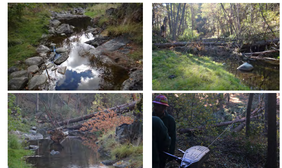
Looking downstream at project site and California Conservation Corps using a grip hoist and cable to move dropped trees on the Cottonwood Creek Accelerated Wood Recruitment Project Phase II.
