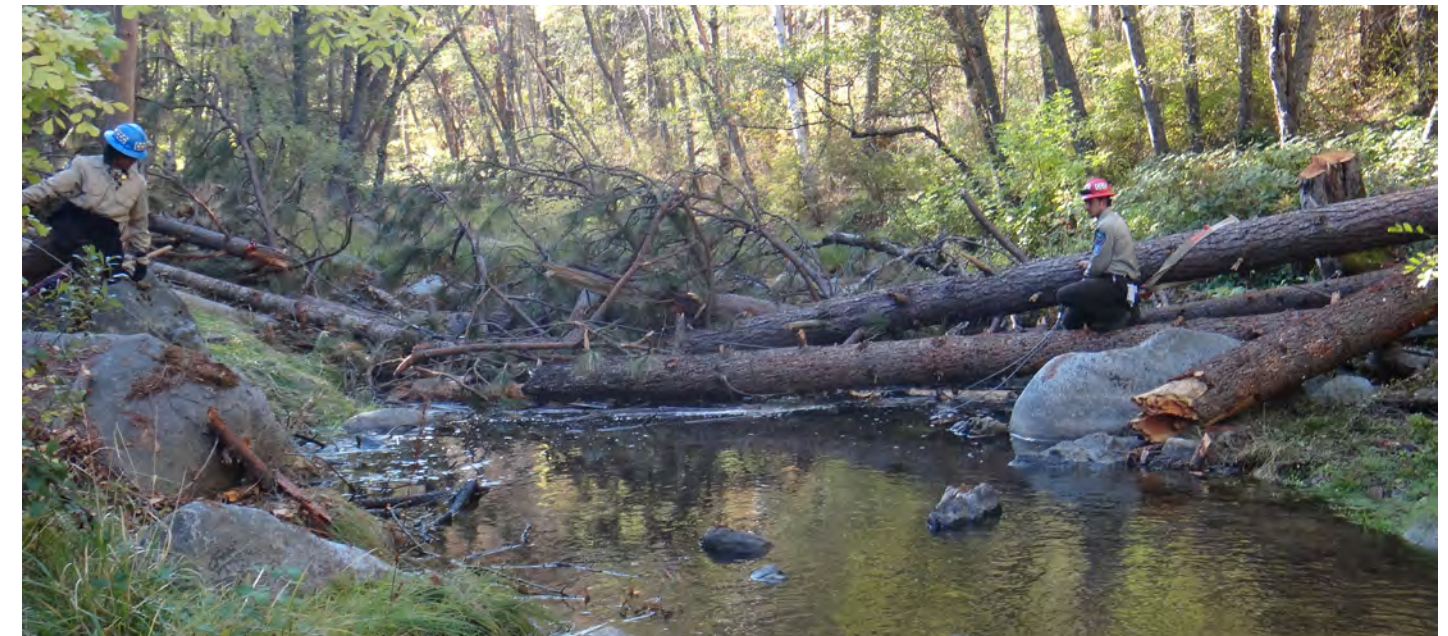
California Conservation Corps constructing Log Jam 2 on the Cottonwood Creek Accelerated Wood Recruitment Project Phase II. ©USFWS.
