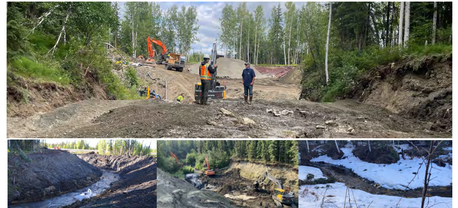
Happy Creek channel construction (top), active construction of stream channel (bottom left), site construction prep (bottom middle), Happy Creek fishway now connects to Cripple Creek natural channel (bottom right). ©USFWS.
