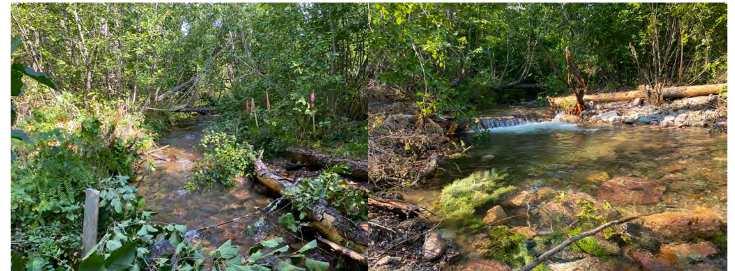
Johnson Creek, pre-fish-screen installation, looking upstream from the irrigation diversion (left). Post-fish-screen installation, looking upstream from the irrigation diversion. The fish screen is visible as a white, underwater shape on river right (right). ©USFWS.
