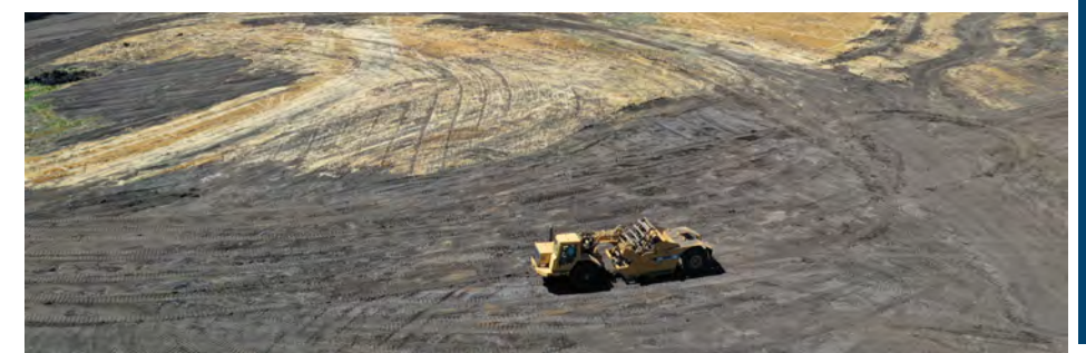
Wetland construction with refuge owned equipment operated by PFW staff. © Matt Blakeley-Smith.
