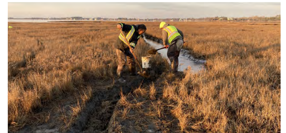
Contractors hand-digging a runnel at Rum Pointe. Photo by Katherine Stahl, USFWS.
