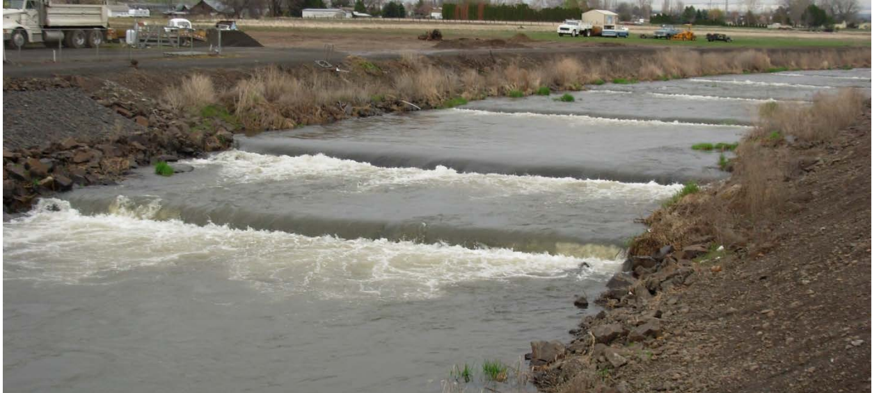
Figure 3.57. Stabilization sills in reach MC20 in lower Mill Creek near Walla Walla, WA.
