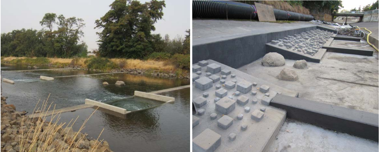
Figure 3.73. Improvements to fish passage in reach MC17 (left) and channel roughness/passage revisions within the concrete flume in reach MC19 in Mill Creek near Walla Walla, WA.
