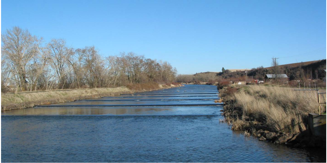
Figure 3.61. Stabilization sills within reach MC17 in Mill Creek near Walla Walla, WA.
