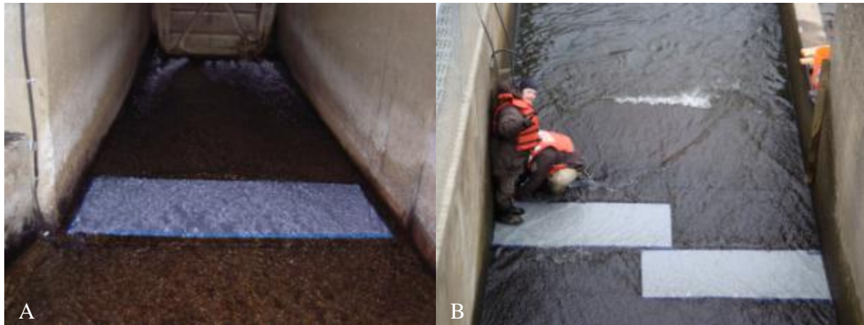
Figure I-13. Low flow outlet showing the original flat plate antenna (A) and two additional flat plates installed just downstream (B).
