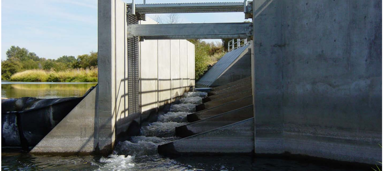
Figure 3.49. Garden City-Old Lowden #2 Diversion Dam and associated fish ladder in reach WW11.
