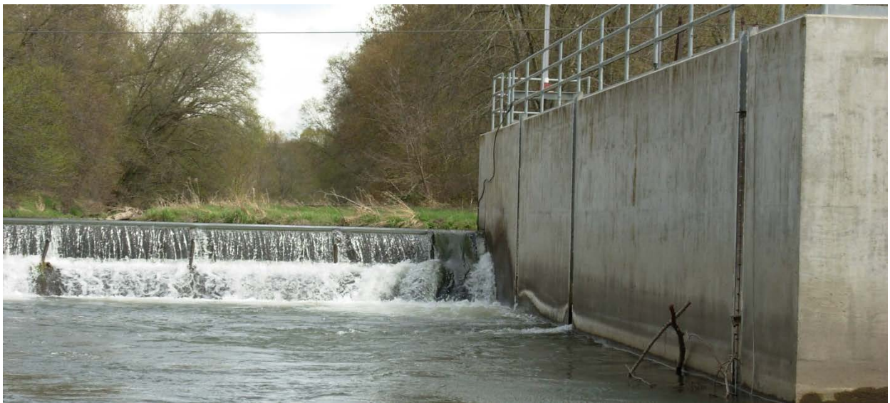
Figure 3.50. Burlingame Diversion Dam and associated fish ladder at the upstream boundary of reach WW10.
