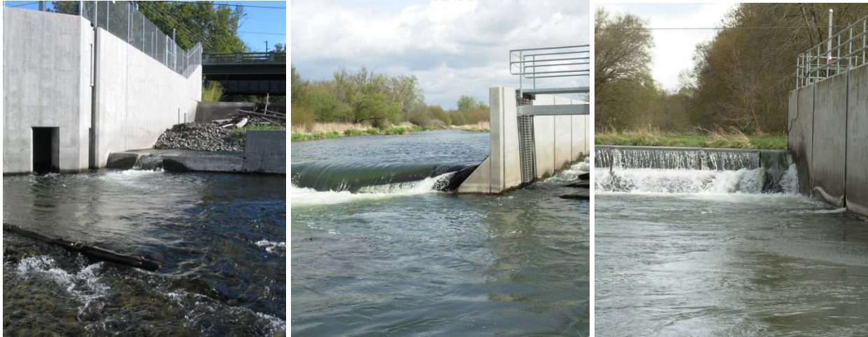
Figure 3.66. Examples of pool-type habitat created by water control structures and diversion dams in middle and lower basin areas. Pictured are Nursery Bridge Dam (left), the Garden City-Old Lowden #2 diversion dam (center) and the Burlingame diversion dam (right) near Milton-Freewater, OR and Lowden, WA.
