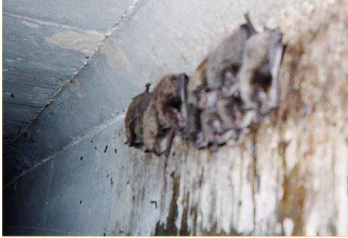
Photo 1: Bats hanging from cracks along support beams
