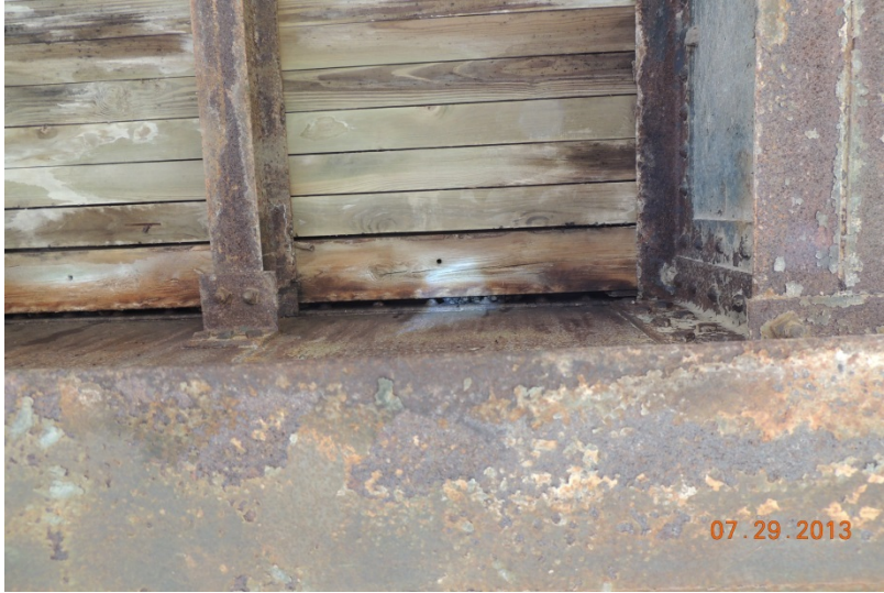
Photo 14: NLEBs roosting under a timber decked bridge
