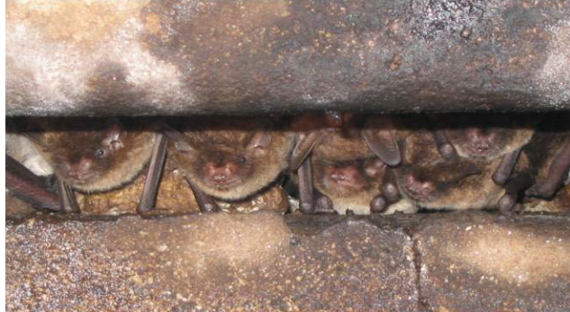
Photo 2: Visible bats within an expansion joint
