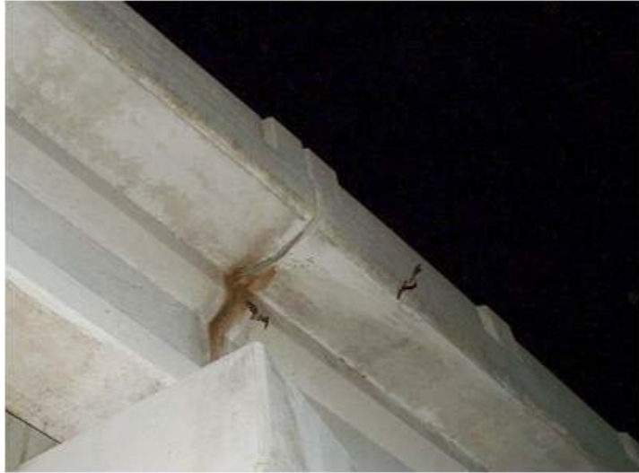
Photo 8: Staining on underside of expansion joint from bat use.
