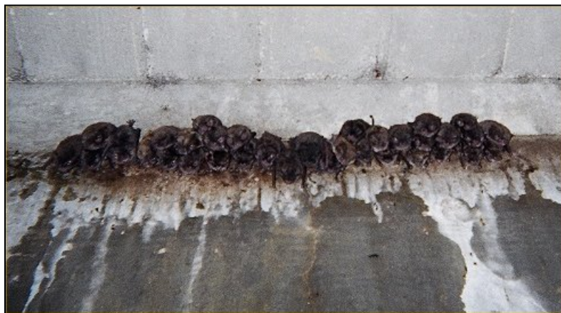
Photo 11: Bats roosting & associated staining
