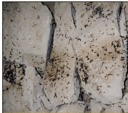
Photo 6: Bat Guano on Riprap
