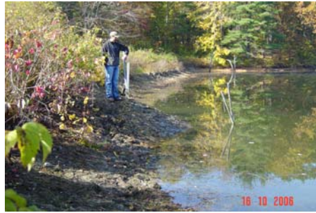
Primary drain plugged
